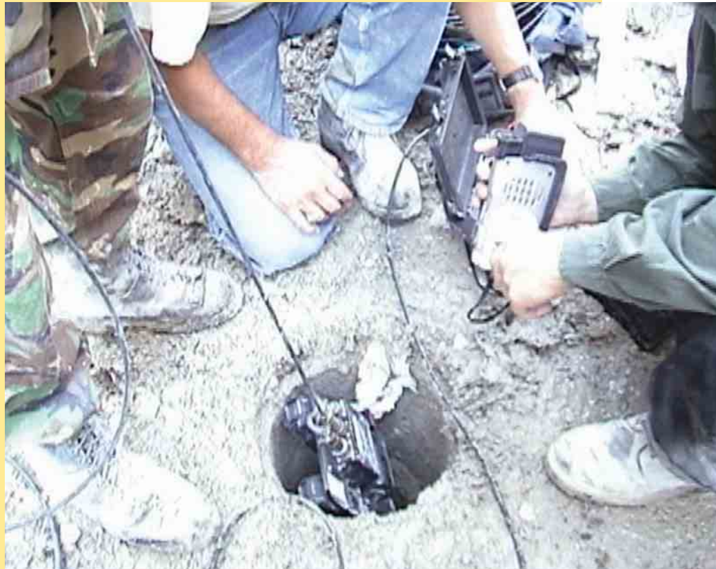
A view of the Inuktun micro-VGTV robot being inserted into a sewer pipe at the World Trade Center site in an attempt to locate an entry to the basement. Note the small size of the robot, the use of a tether as a safety line for the vertical entry, and the use of a camcorder to display the video because of better resolution than the manufacturer's display. This is the only external view of the robots entry that was allowed to be photographed at the WTC site.
